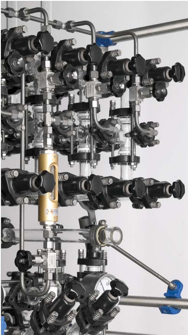
Precise manufacturing allows complex installations in small space
